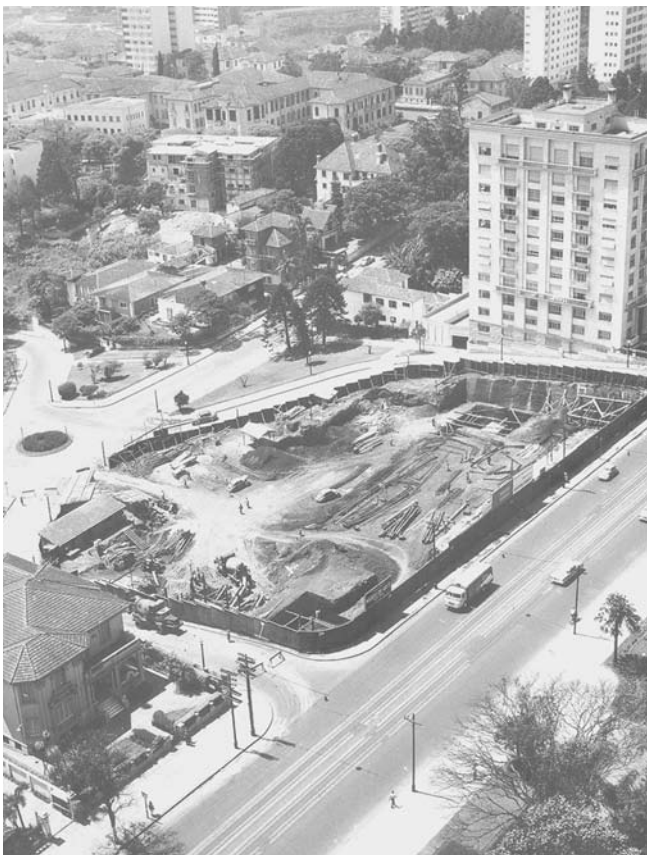
LEFT: Trianon Terrace site after demolition and during the construction of the foundations for the new Museum of Art of São Paulo in the early 1960s.
